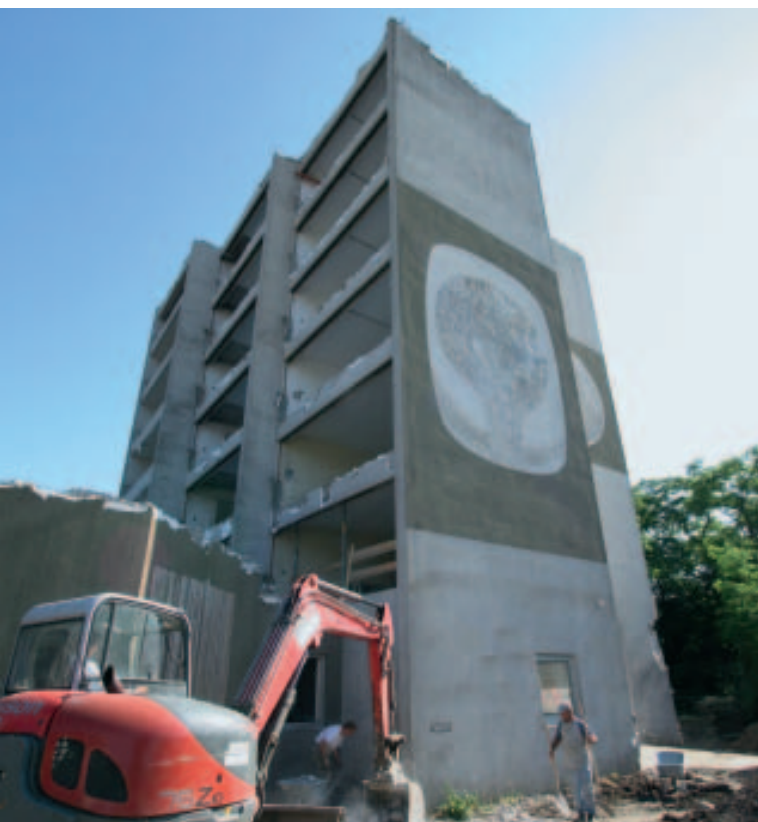
Gutted down to the bare walls: the "St. Koloman – House of Generations" before its renovation.
